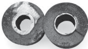
The cross section of the coil on the right shows how internal corrosion caused by improper piping, trapping and venting may destroy coils from the inside out.
